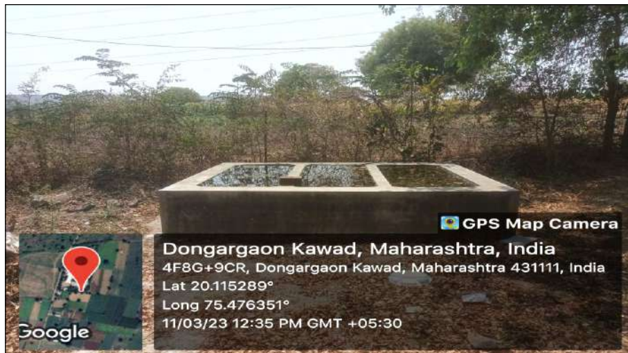
Water Tank for Algae
